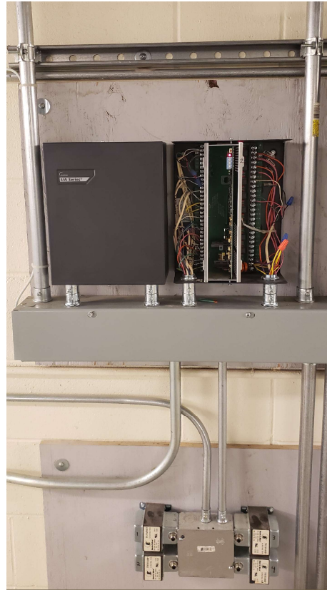
Necessary upgrades to HVAC controls
