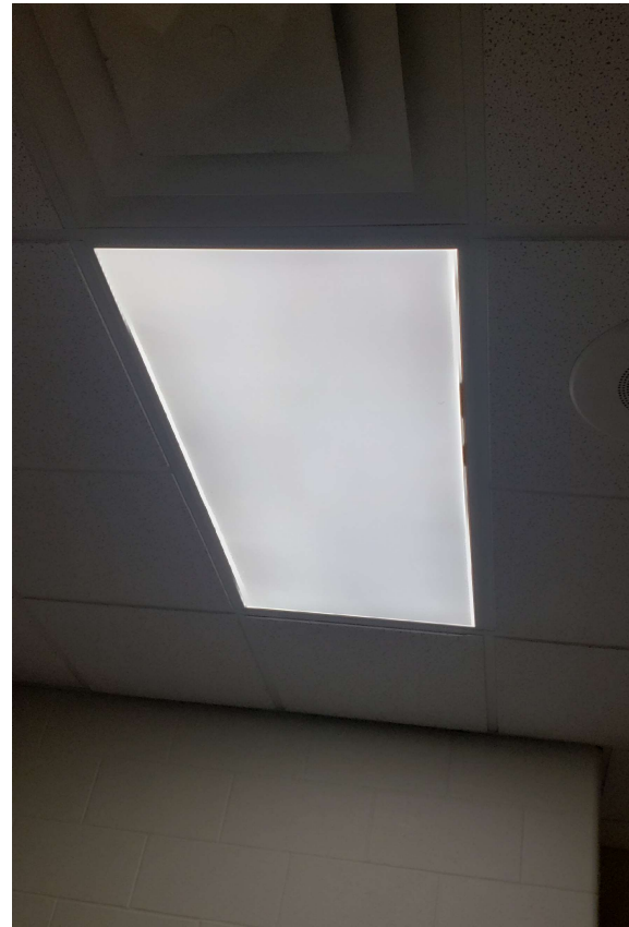
New LED lighting
