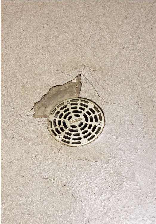
Epoxy repair needed
